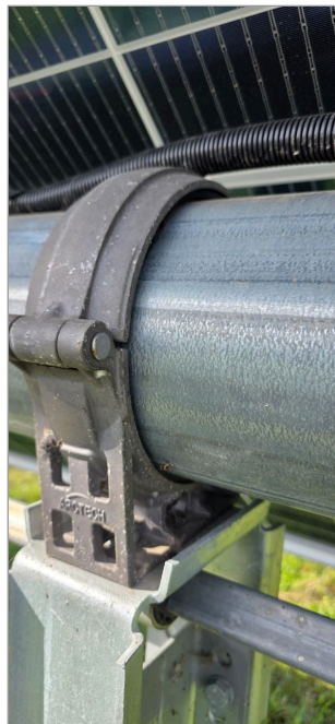
Figure 4 — 17 August 2026. A second position, inspected six days later: same condition.
